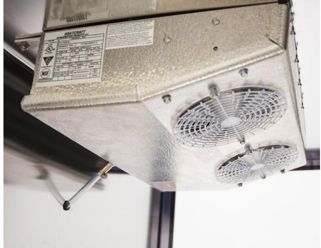
Figure 18: Drain tube exiting the evaporator inside the pass-through
